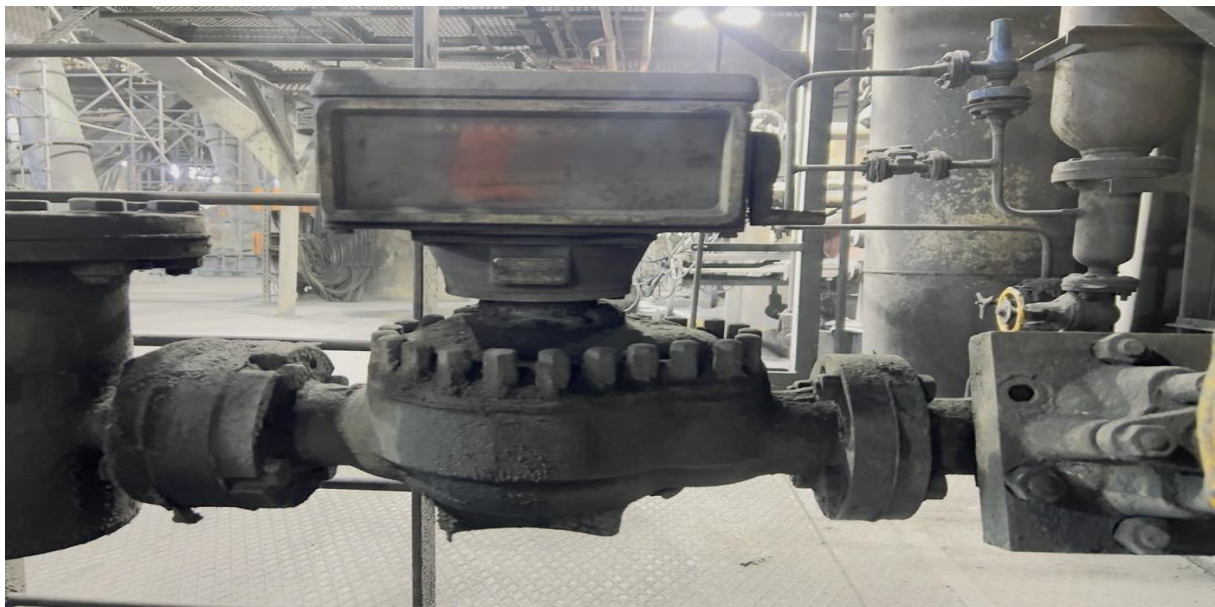
Figure 3: Unit 2, 4, and 5 flow meters to be replaced
