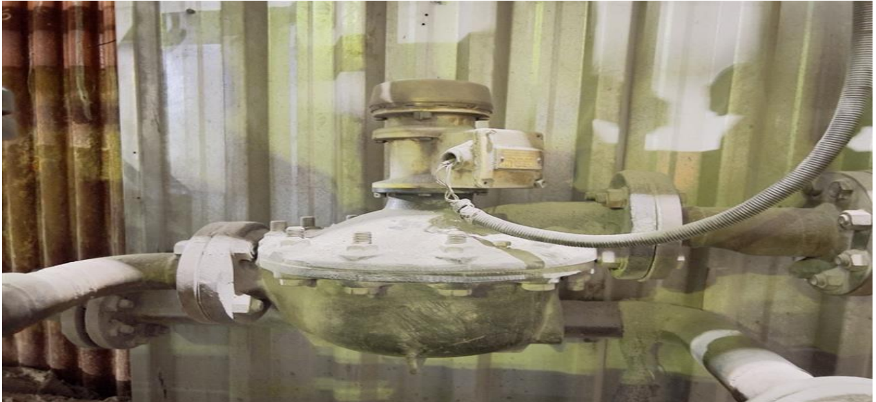
Figure 2: Units 6, 7, and 10 flow meters to be replaced
