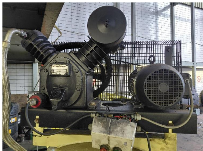
Picture 2: Two stage compressor unit.
