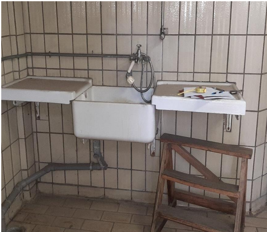
Figure A.6: NMC battery room sink.
