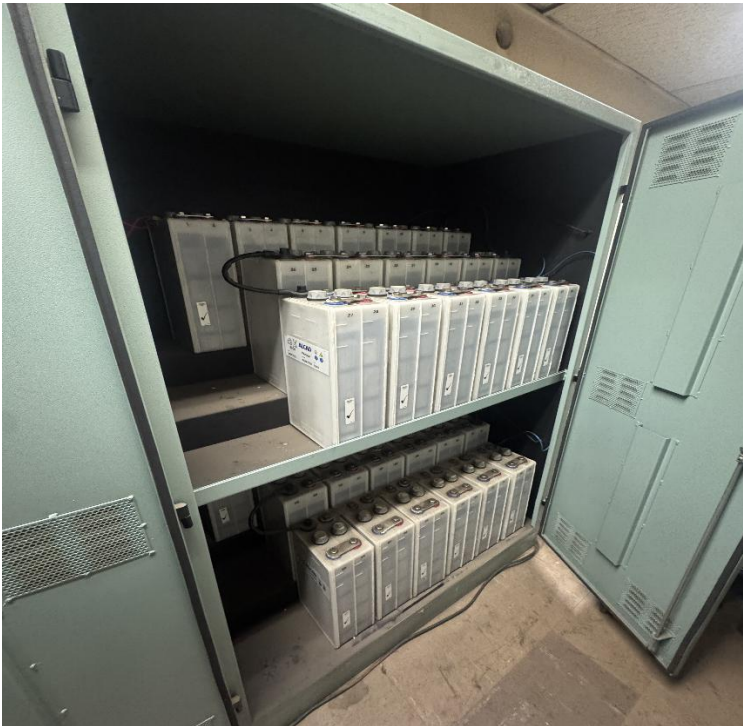
Figure A.8: NMC Charger battery bank (38//38)
