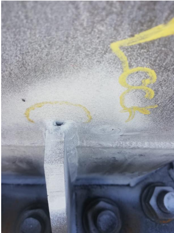
Photo 13: Weld defect at stiffener
