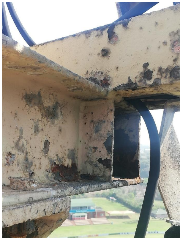
Photo 16: Corrosion on web of cross-arm support
