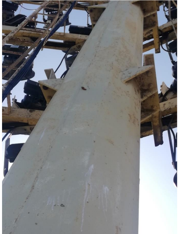
Photo 22: Corrosion on cat ladders
