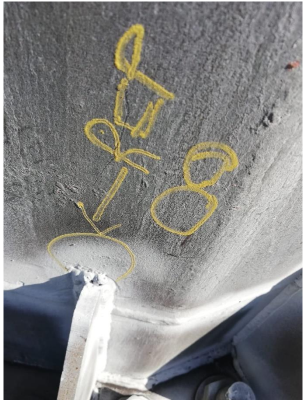
Photo 14: Weld defect at stiffener
