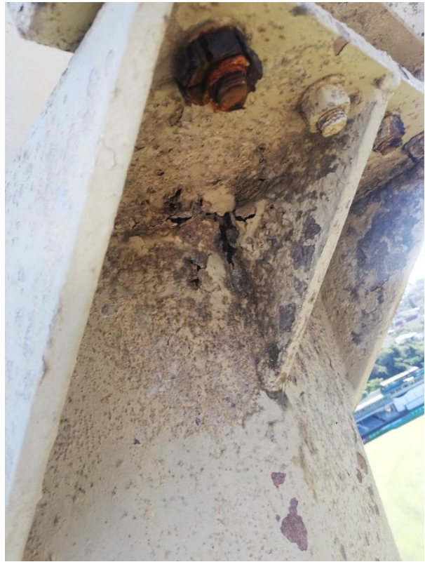
Photo 18: M1 – Corrosion of nut
