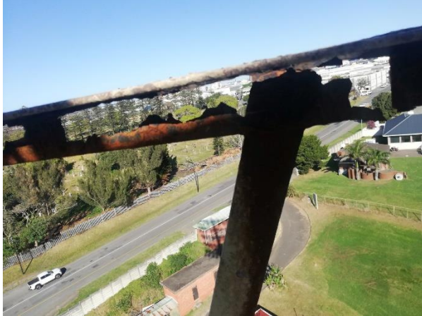
Photo 21: Corrosion of handrail
