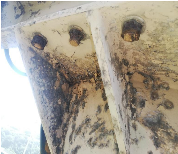
Photo 23: Corrosion on nuts
