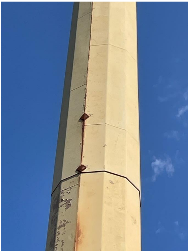
Photo 12: M4 - Corrosion on weld strengthening plates
