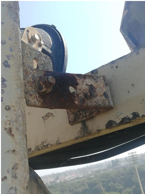
Photo 15: Corrosion on cross-arm attachment
