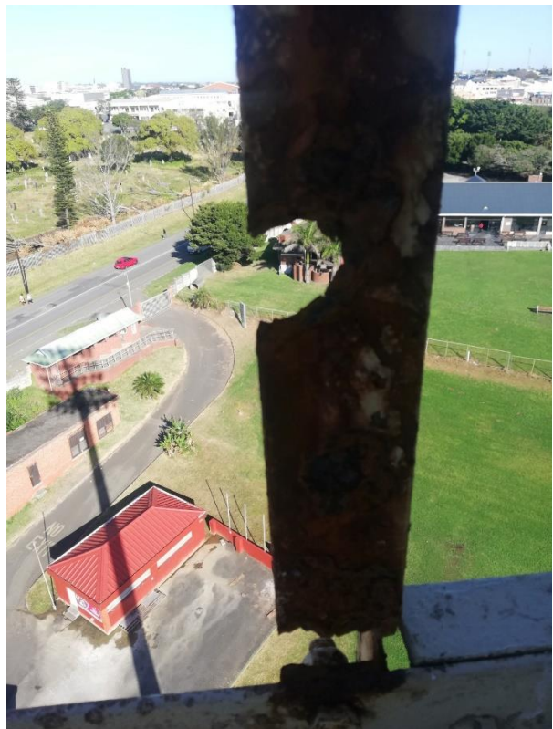
Photo 20: Corrosion on handrail vertical
