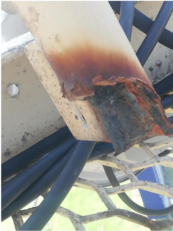
Photo 17:M1 – Corrosion on member
