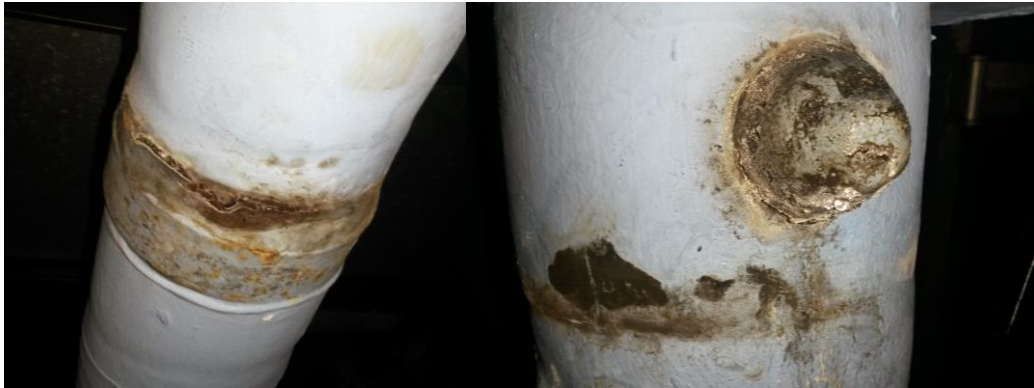
Figure 13: Damaged chilled water piping insulation as for Plantroom 7 units
