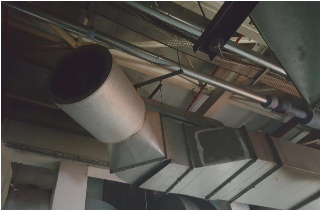
Figure 24: Toilet Exhaust duct with no fan in Plantroom 2
