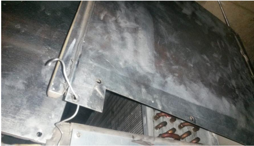
Figure 8: Kenya Airways Offices – FCU missing panel bolts
