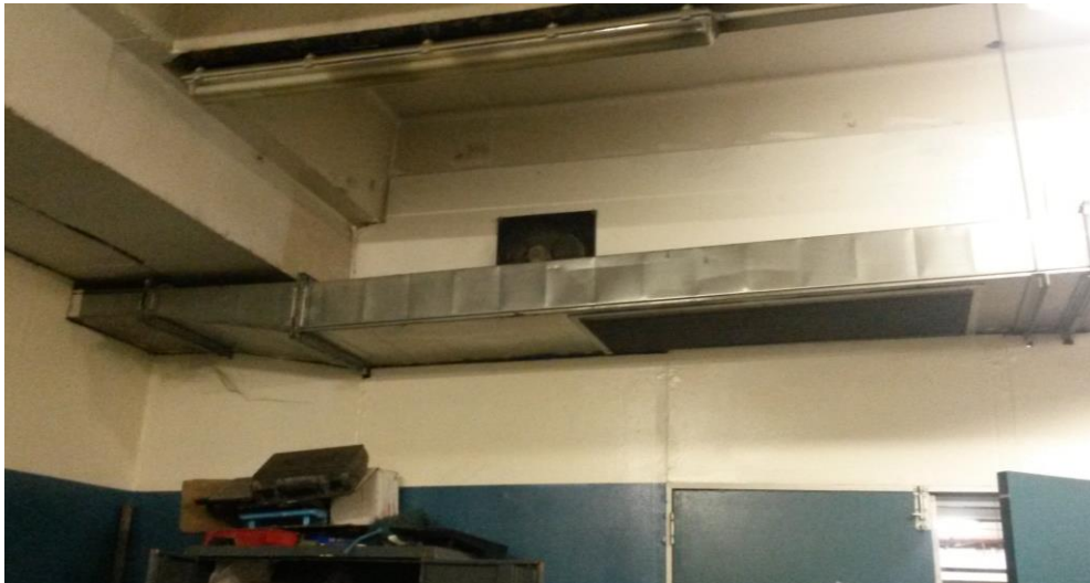
Figure 5: Crisplant Mechanical Workshop - the small wall mounted fan semi blocked by the passing duct
