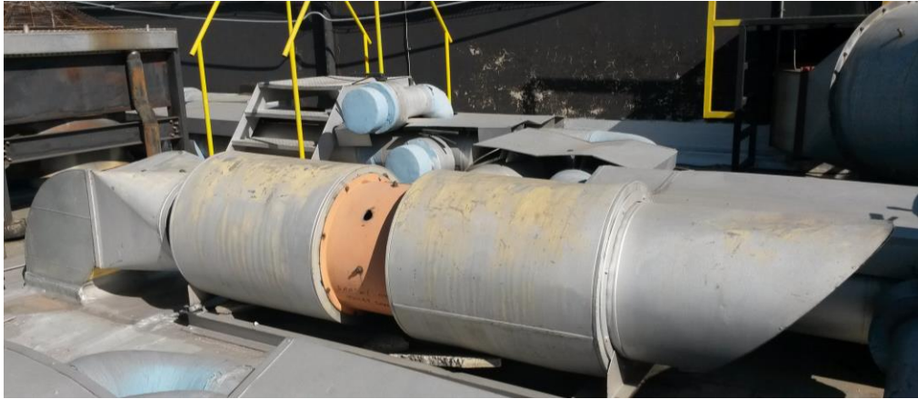
Figure 18: Toilet Exhaust Fan - Ducting dented
