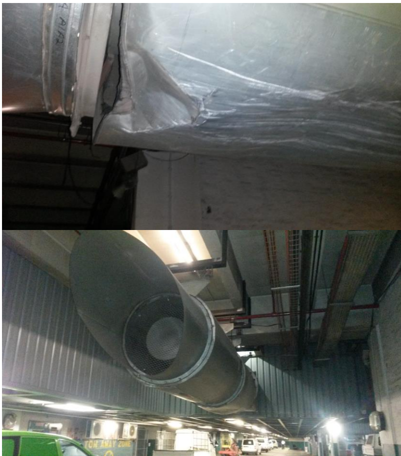
Figure 2: The damaged ducting of the large exhaust fan
