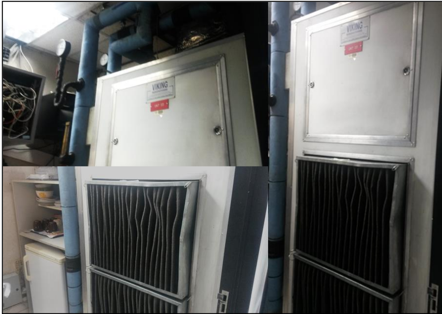
Figure 11: TAAG Offices - AHU 115 in same space as occupants' kitchen area
