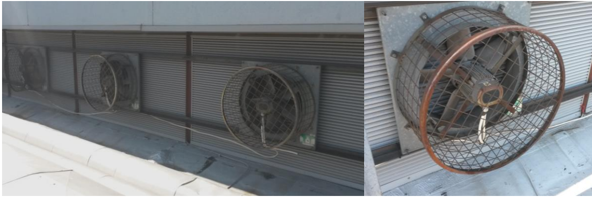
Figure 23: Fans mounted to weather louvres serving the Viewing Deck on the Lower Roof Level
