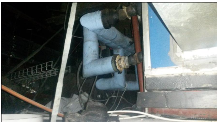
Figure 10: UTS Store Room - FCU Chilled Water pipping condition
