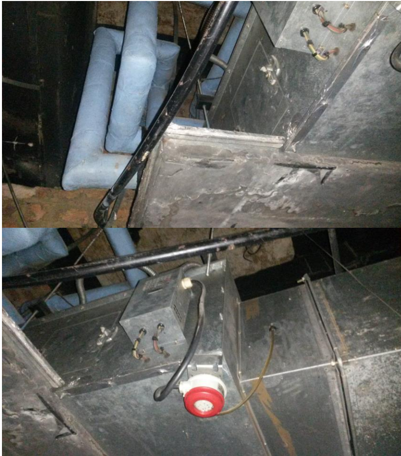
Figure 7: FCU 79 supplying the Police Station Office
