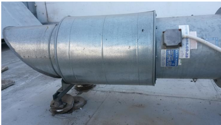
Figure 17: Toilet Exhaust Fan - Leg support of fan
