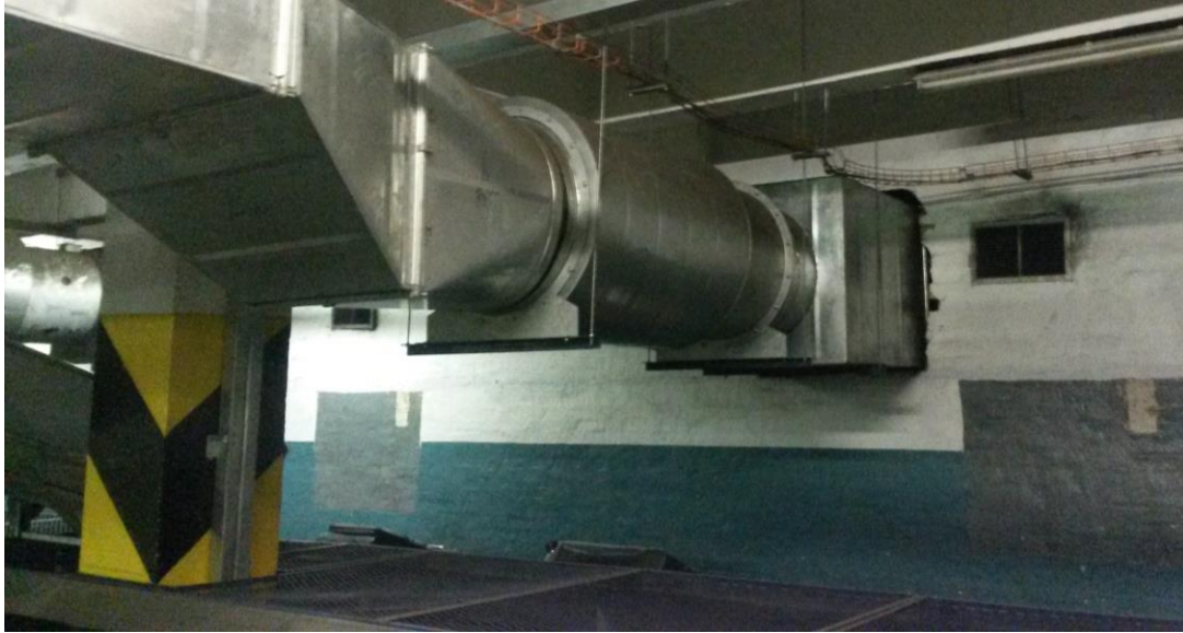
Figure 4: Basement exhaust fan - BB1 as labelled on site
