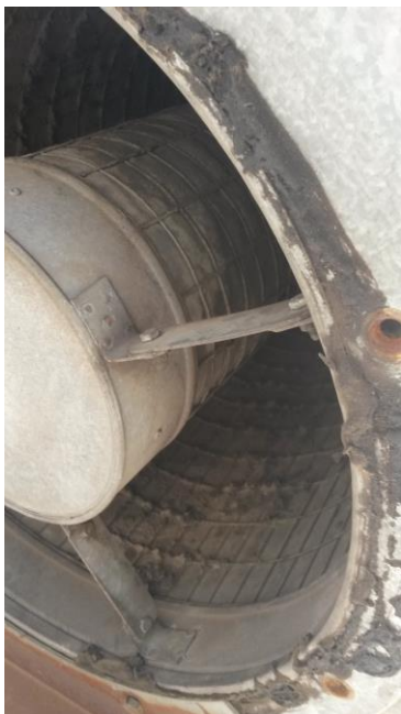
Figure 20: Toilet Exhaust Fan with no mesh at exhaust air exit
