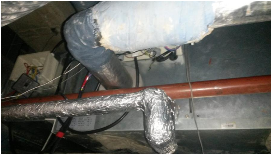
Figure 9: Kenya Airways Offices – FCU Chilled Water pipping and Electrical Wiring condition
