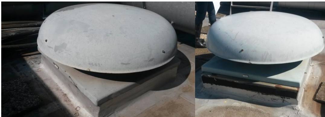
Figure 16: Example of a typical Roof Fan
