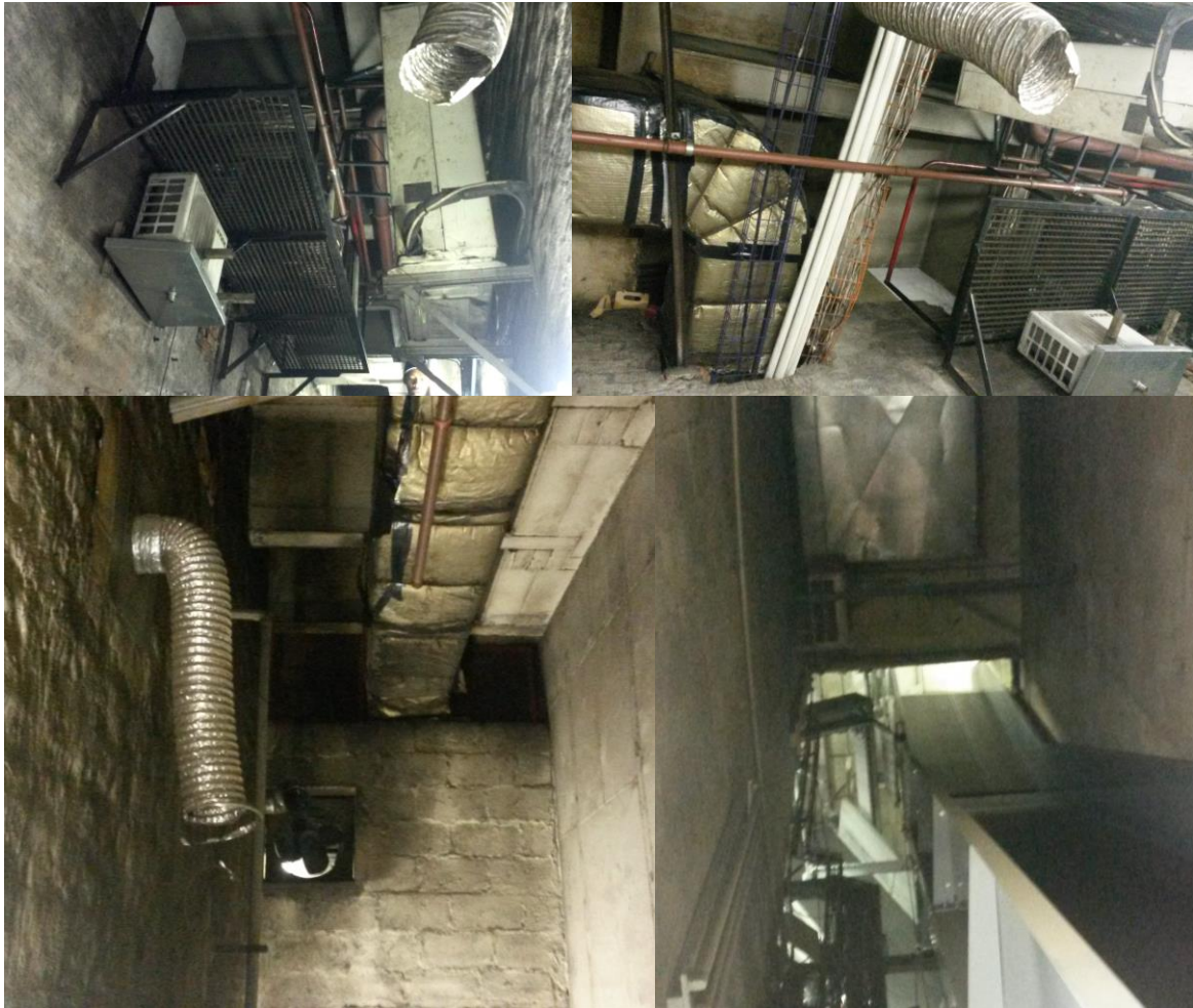
Figure 6: Baggage carousels connecting level shafts - all HVAC equipment not in use anymore
