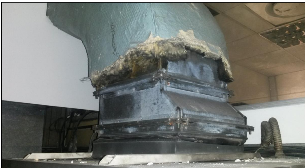
Figure 12: FCU xx (GL 33-34 & I-J) in office room acting as plantroom
