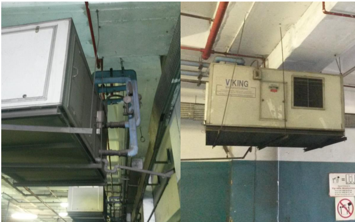
Figure 3: Un-ducted FCU suspended from the ceiling slab in the Baggage Handling area of the basement
