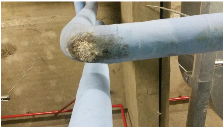
Figure 14: Damaged chilled water piping insulation for Plantroom 8 units
