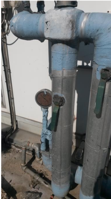
Figure 15: Example of Chilled Water Piping condition of AHU 121
