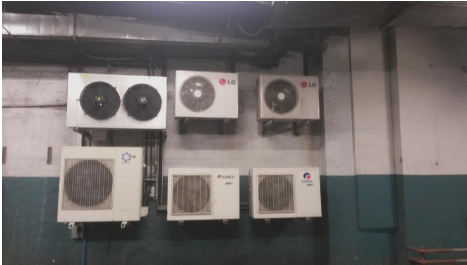
Figure 1: Example of Split Outdoor Units – Condensers
