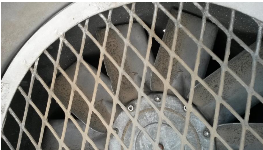
Figure 22: Toilet Exhaust Fan - example of blade condition
