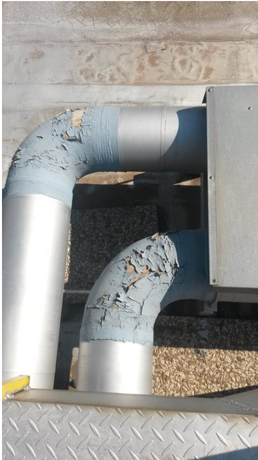
Figure 21: Example of Chilled Water Piping insulation cracked at an elbow bend
