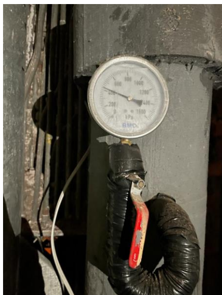
Figure 3: Chilled Water pressure gauge reading
