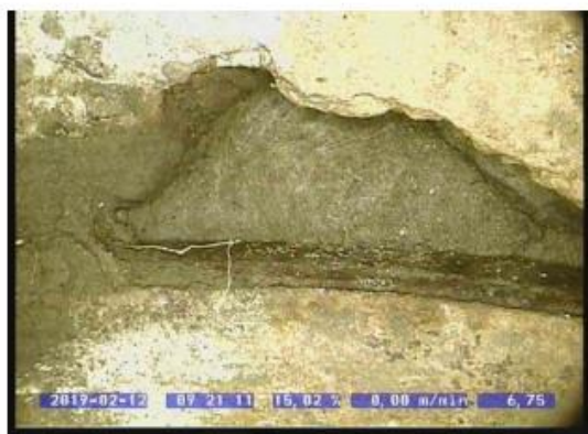
IB924IB923_5148e35b-5f3e-4467-bbb3-cbe76bf29c74_20190212_092633_465.jpg, 00:02:10, 6.75m Broken pipe at joint from 10 o'clock to 11 o'clock ,
