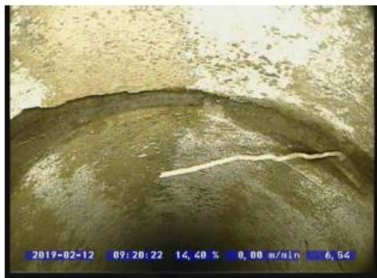
IB924IB923_a68075e8-99a3-4a0e-8689-9c6a0a549afd_20190212_092544_581.jpg, 00:01:21, 6.54m Roots, tap at joint
