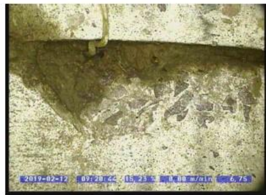
IB924IB923_521d0a29-fe39-406b-ac6a-29c8abb10171_20190212_092607_409.jpg, 00:01:44, 6.75m Broken pipe at joint at 3 o'clock ,
