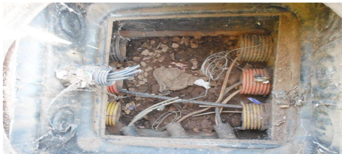
FIGURE 4.2.2: VANDALISED MANHOLES ON PLATFORM CABLE WIRING
