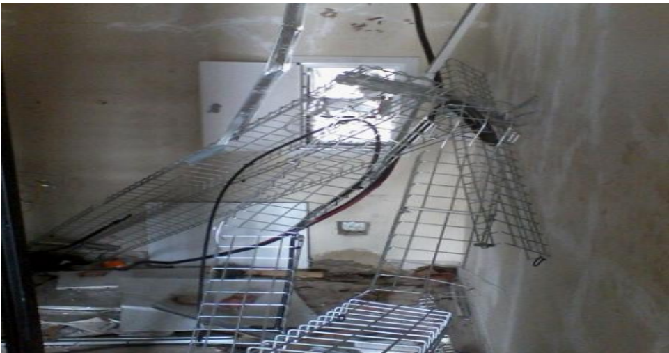
FIGURE 4.2.4: VANDALISED CABLE TRAYS
