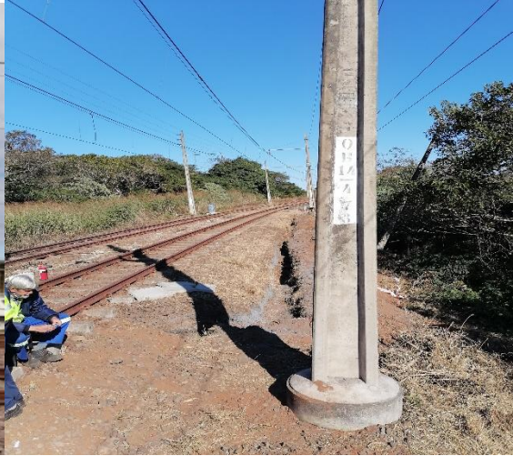
Figure 2: shifted Pole at Umbongintwini
