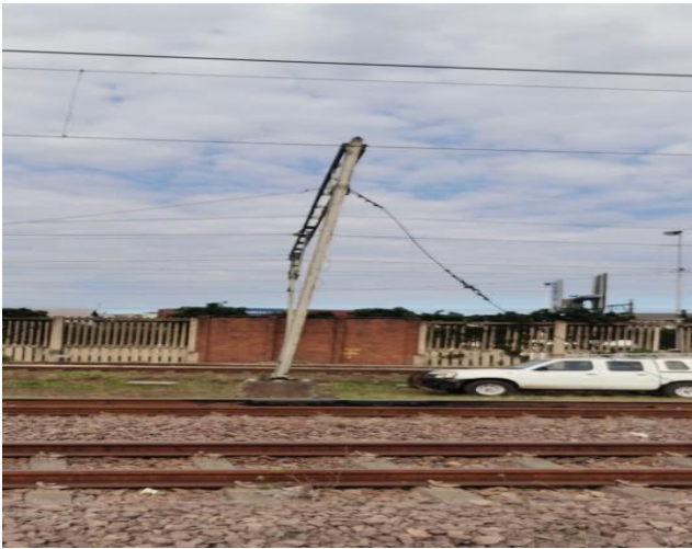
Figure 1: Bent Mast Pole at Congella
